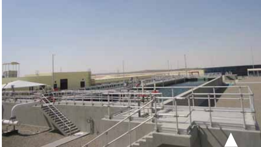
Razeen Sewage Plant, Abu Dhabi, UAE
