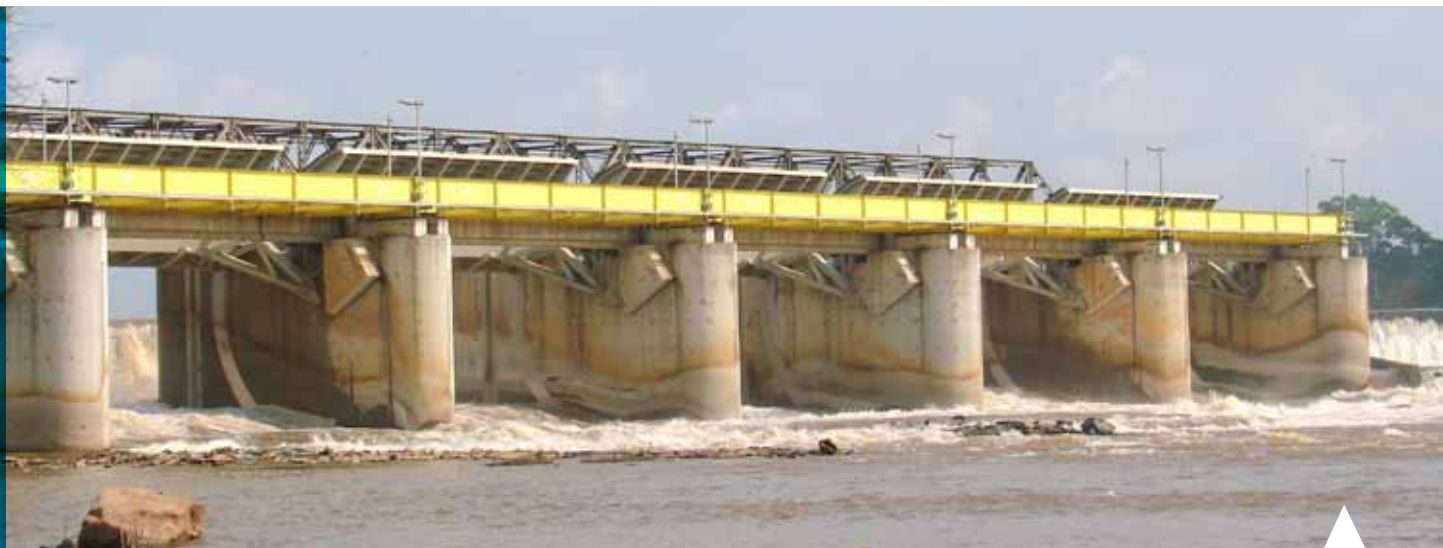
Edea Spillway, Edea, Cameroon
